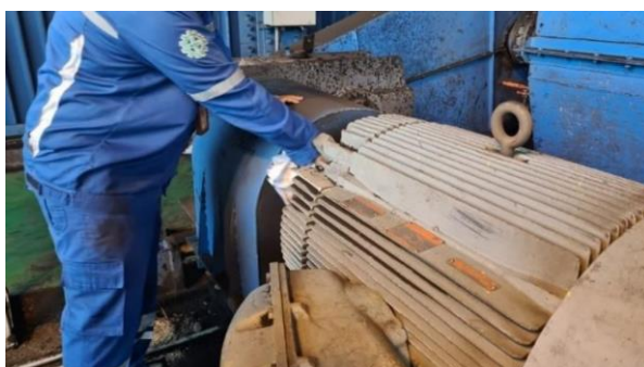
Figure 6 Routine conveyor motor cleaning
